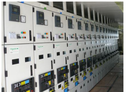
Schneider Electric Switchgear Installation
