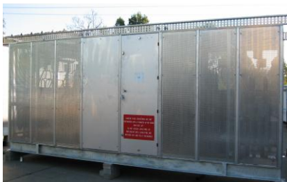
Tea Garden High Voltage Unit A1511
