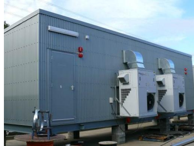
APLNG Switchroom Building 8110
