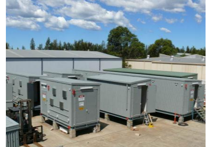
APLNG Switchrooms Complete
