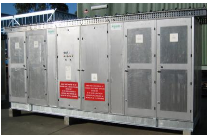
Tea Garden High Voltage Unit B 1512
