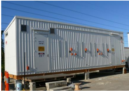
QAL Control Room 0897
