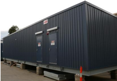
ABB Joe White Switchroom 0916
